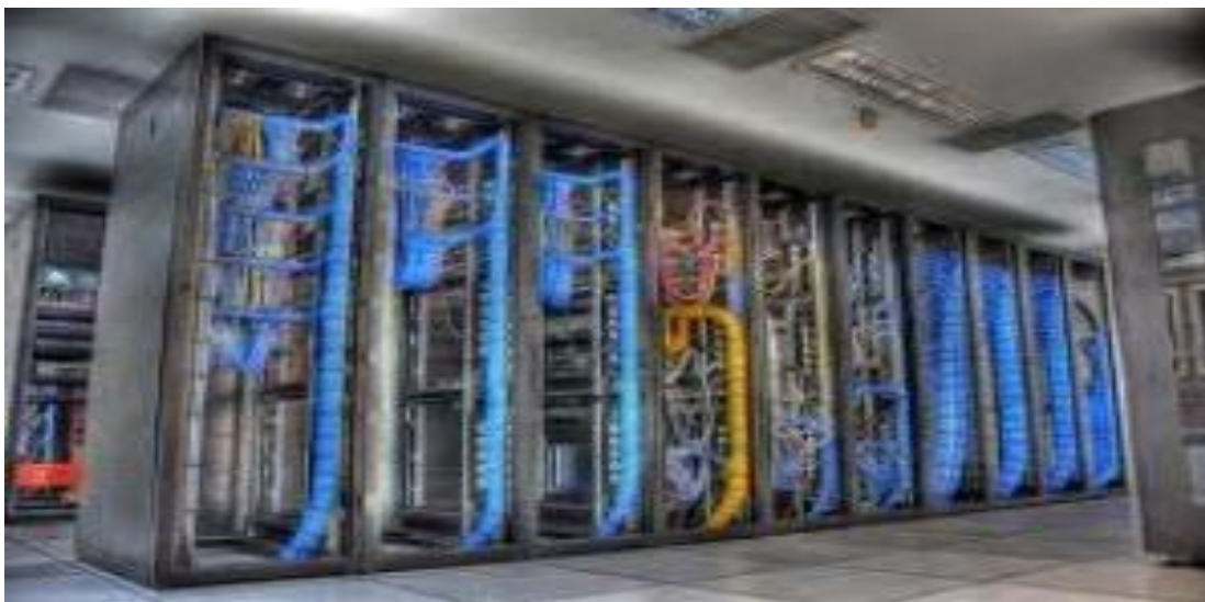
Figure 2.8: Structured caballing of a data center
